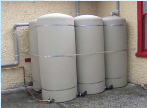
Water tanks at the YWCA supply bathrooms whilst reducing storm water runoff.
